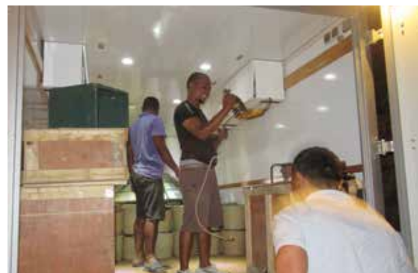
The interior of the ADES north mobile being modified.
