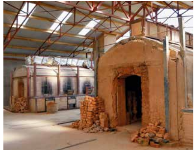
The new oven (at the back) is underground and linked to the other oven.
